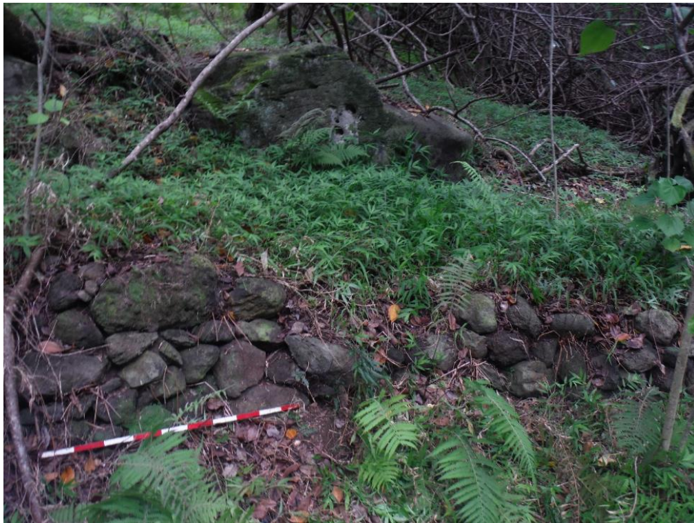
Figure 41. South retaining wall in excellent condition in feature WAI-2-L, view to S.
