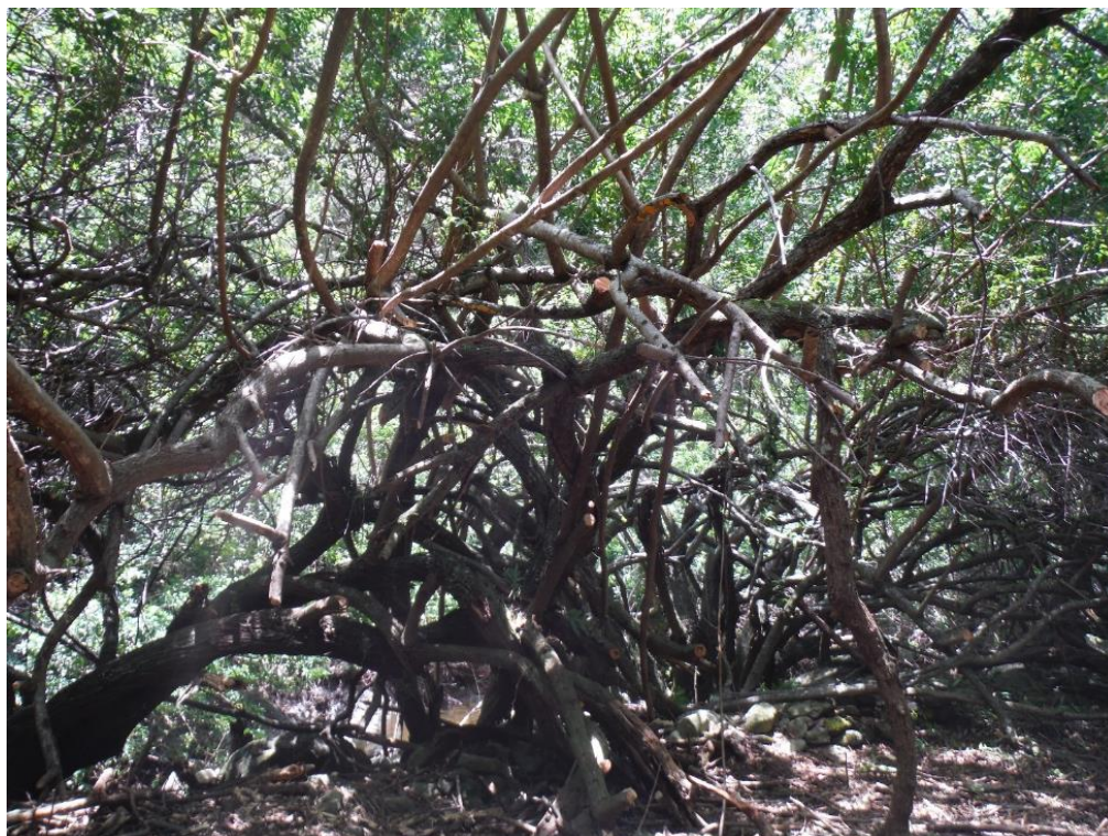
Figure 44. Dead tree canopy in feature WAI-2-U. Note: Tree system is growing within the structure of the retaining wall.
