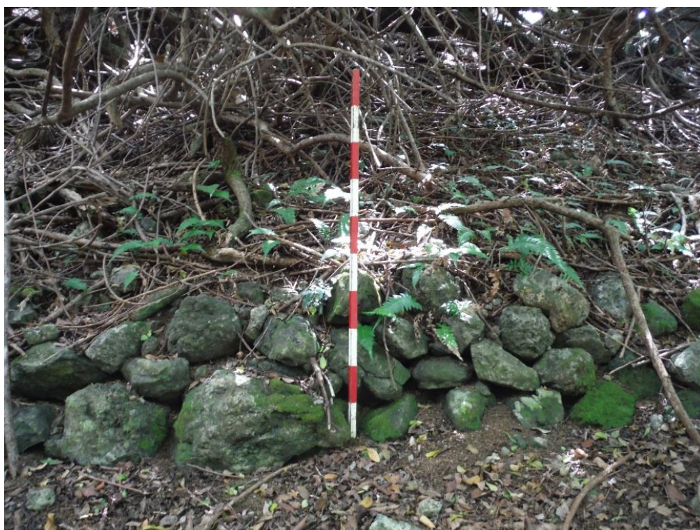
Figure 47. Vegetation overgrowth along West retaining wall of feature WAI-4W-Y, view to W.
