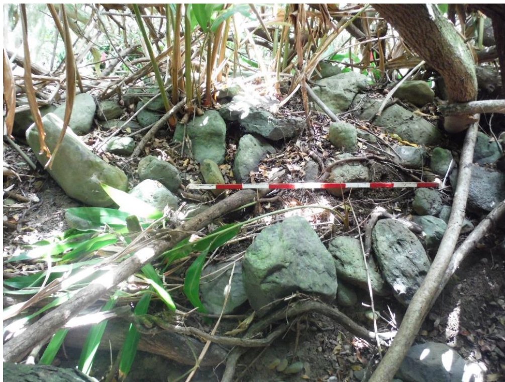
Figure 42. Vegetation overgrowth present in West retaining wall in feature WAI-2-S, view to E.
