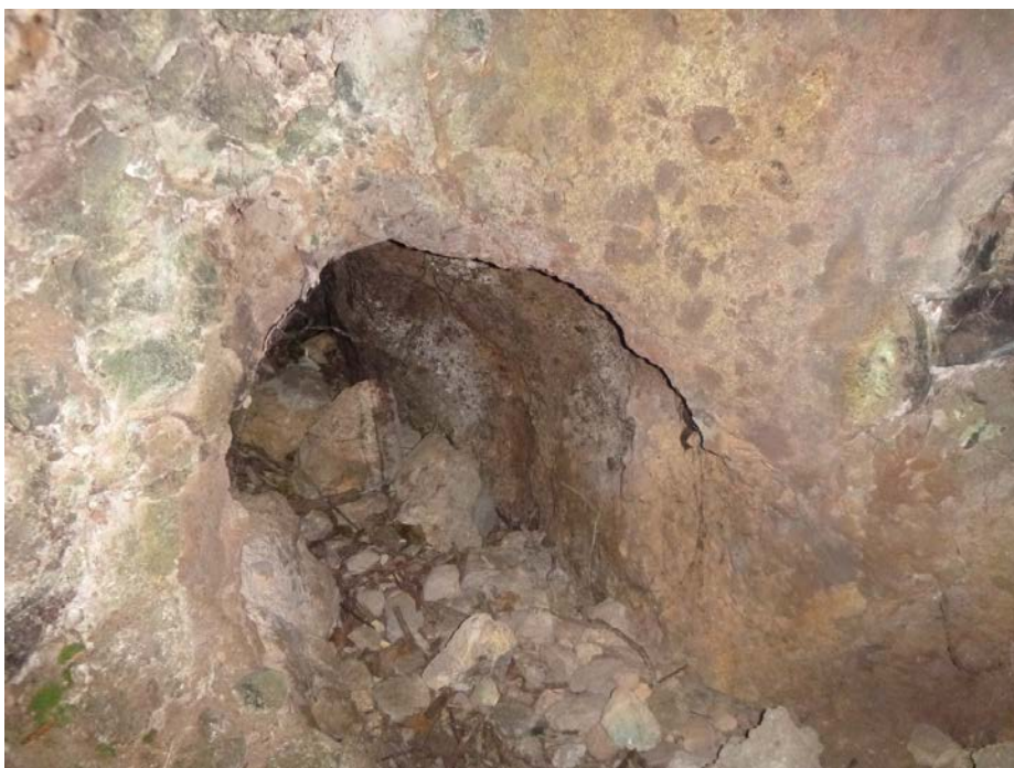
Figure 22. Entry to Wai'āpuka Tunnel showing excavation through bedrock of the tunnel passage way.
